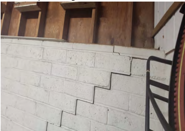
47 Differential Step Cracking Bicycle Storage
