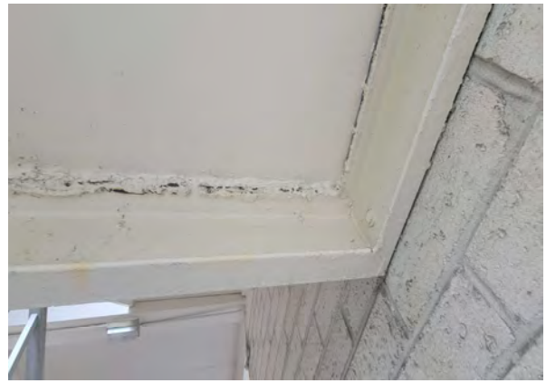
74 Hallway E Rust at Stairs
