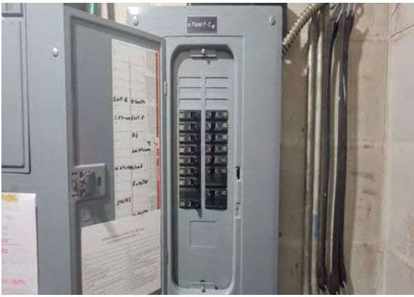
17 Sub Panel Internal
