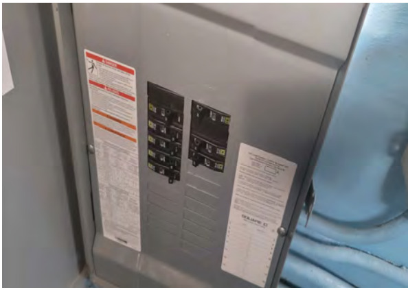
57 Pool Room Electrical Panel Internal
