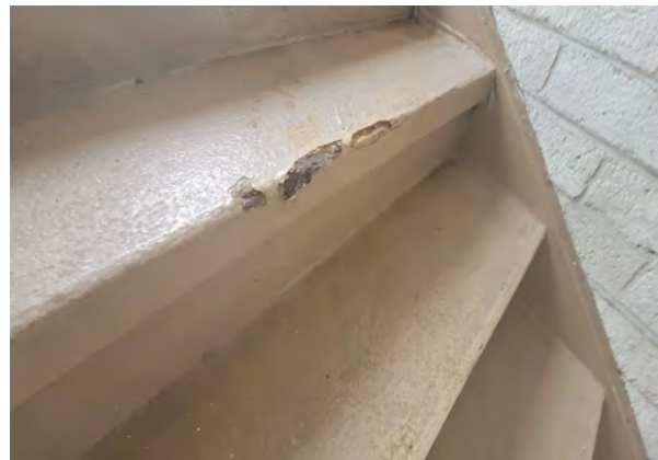
70 Hallway F Rust at Stairs
