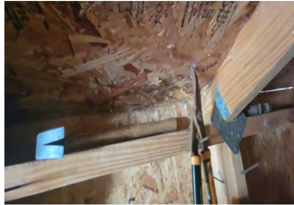
68 Tool Shed Water Penetration
