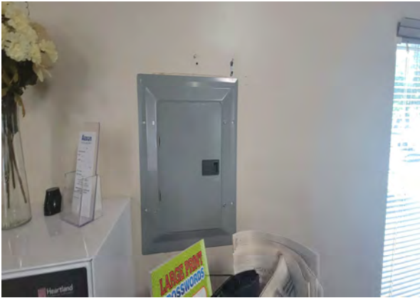
11 Clubhouse Electrical Panel
