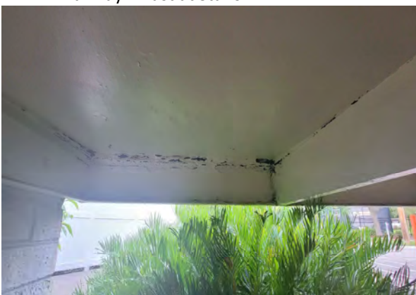
71 Hallway F Rust at Stairs
