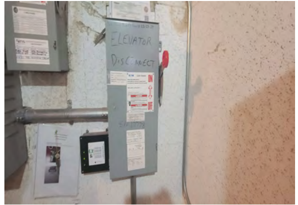
20 Elevator Cab Disconnect
