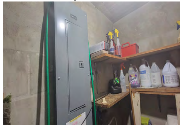
40 Chemical Storage Electrical Panel
