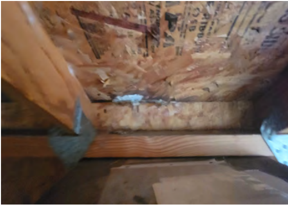
67 Tool Shed Water Penetration
