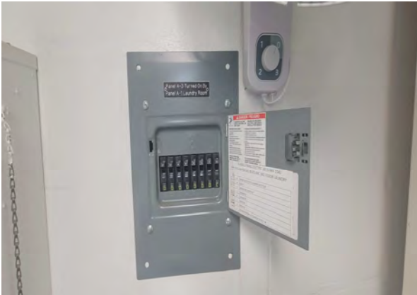
27 Laundry Room Electrical Sub Panel Internal
