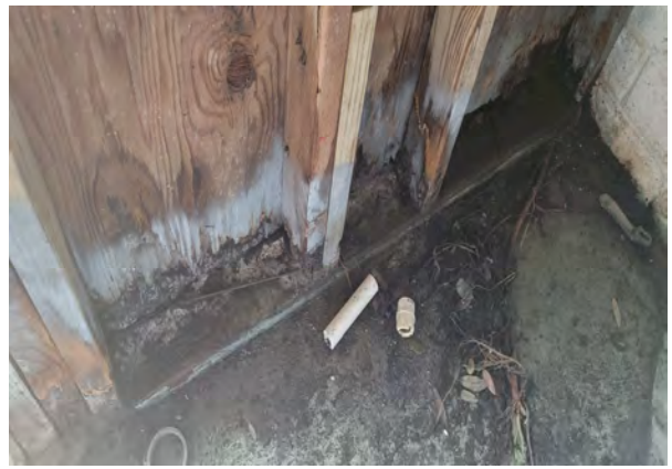
58 Water Damage/Organic Growth Pool Pump Room
