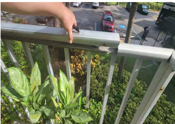
86 Loose Rail Cap
