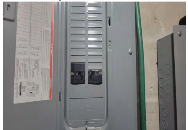
16 Main Panel Internal
