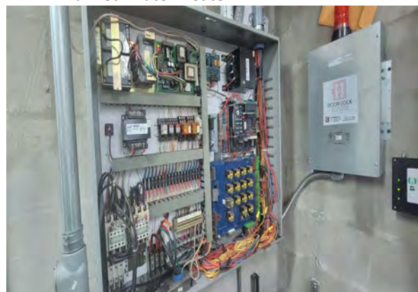
32 Elevator Control Board
