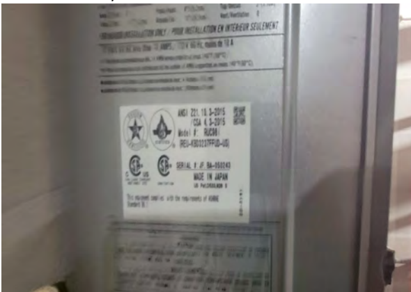
29 Tankless Water Heater Data Label
