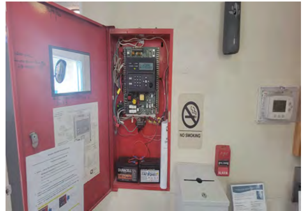
6 Fire Alarm Internal
