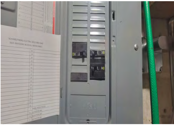
41 Chemical Storage Eletrical Panel Internal
