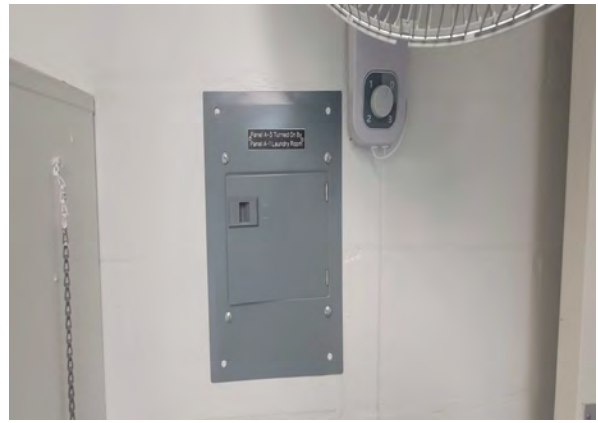
26 Laundry Room Electrical Sub Panel
