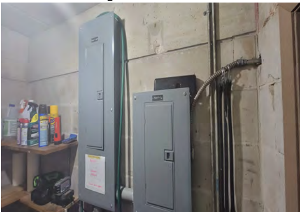
15 Main and Sub Electrical Panels
