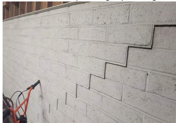
48 Differential Step Cracking Bicycle Storage
