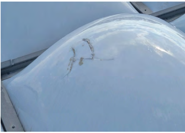
80 Cracks in Skylight
