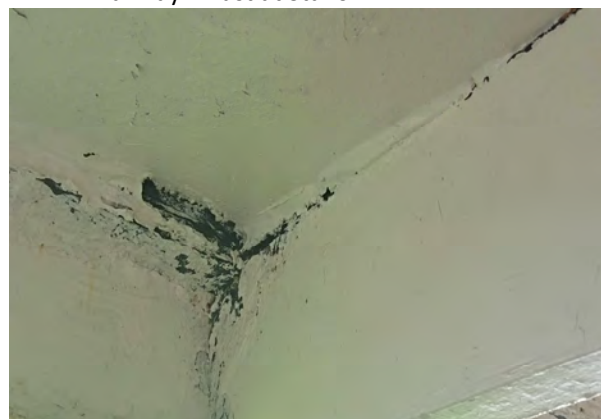
72 Hallway F Rust at Stairs
