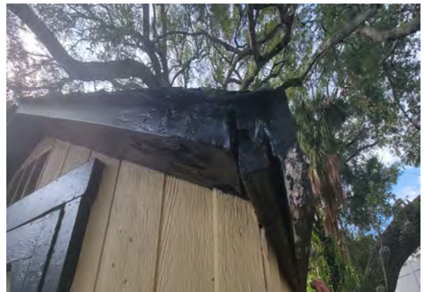
64 Tool Shed Water Damage
