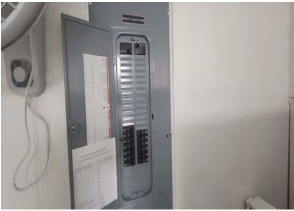
25 Laundry Room Electrical Panel Internal
