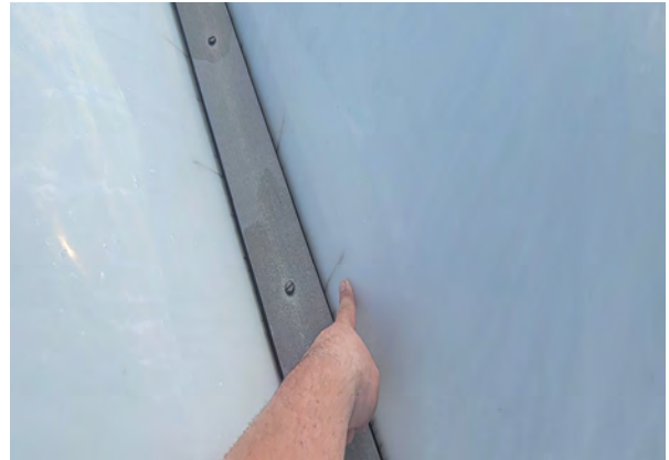
83 Cracks in Skylight
