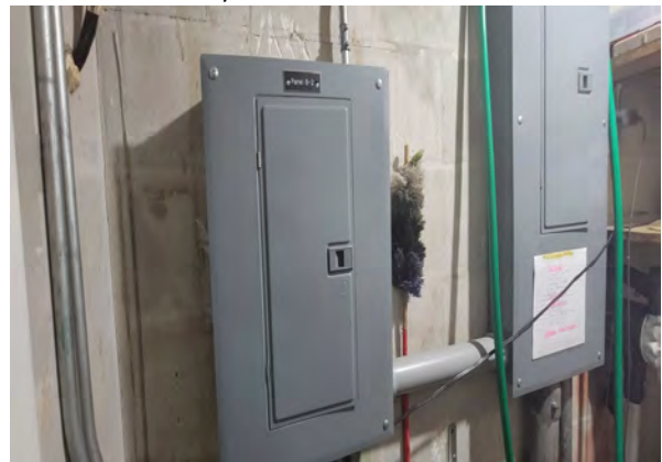
38 Chemical Storage Sub Electrical Panel
