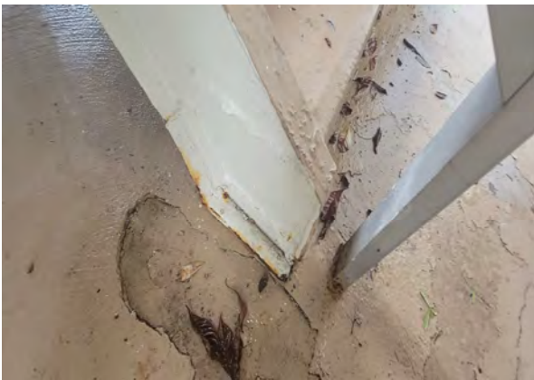
69 Hallway F Rust at Stairs
