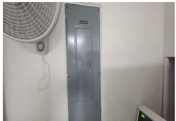
24 Laundry Room Electrical Panel
