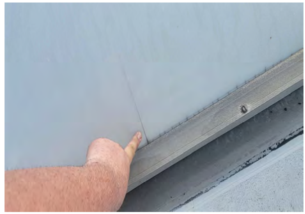
81 Cracks in Skylight
