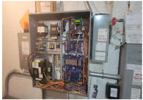
18 Elevator Control Board
