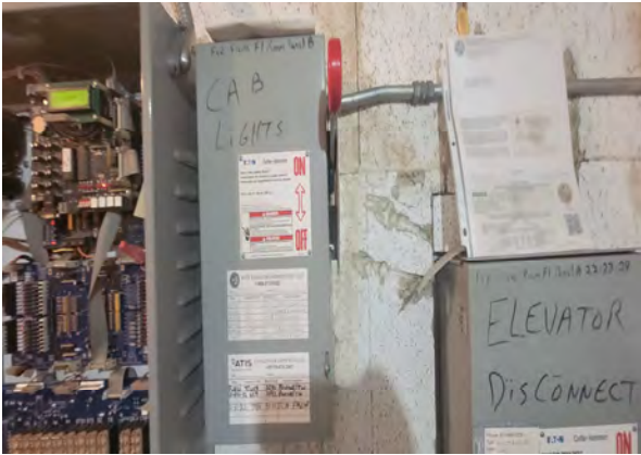
19 Elevator Light Disconnect
