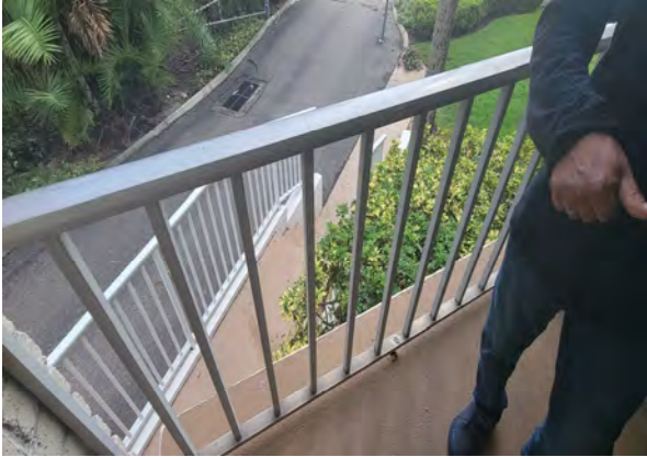
75 Hallway A Stairs Loose Spindles and Rust
