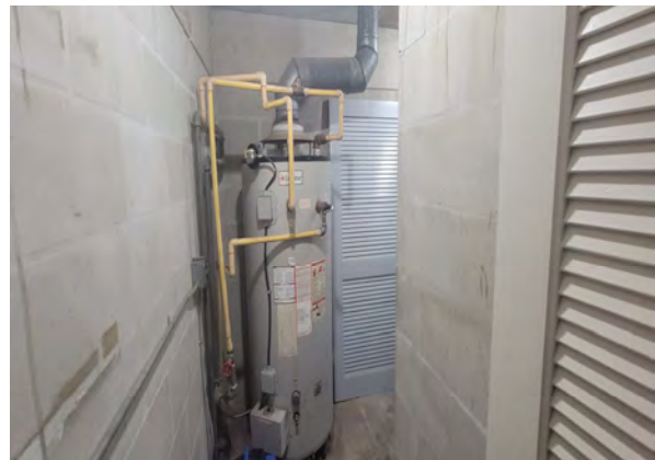
30 Tanked Water Heater
