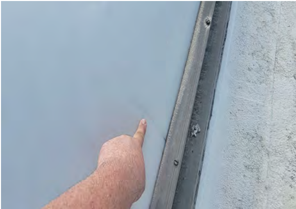
82 Cracks in Skylight
