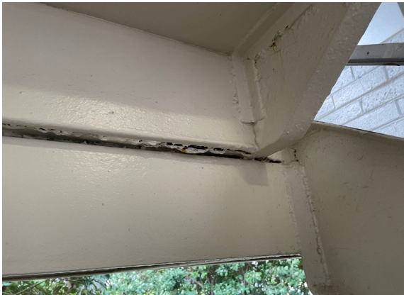
21 stairwell B corrosion
