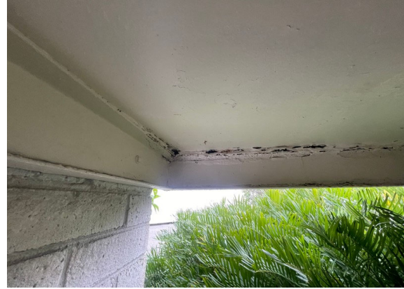
36 stairwell F corrosion
