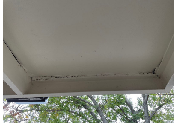
28 stairwell E corrosion
