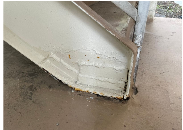
6 stairwell A corrosion
