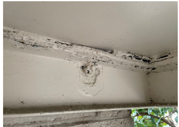
16 stairwell B corrosion
