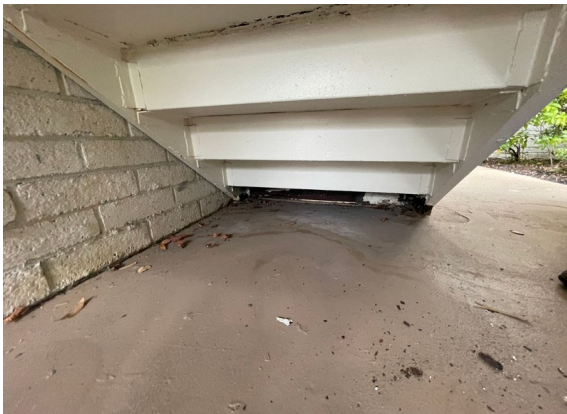
39 stairwell F corrosion
