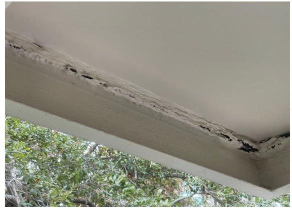
26 stairwell B corrosion
