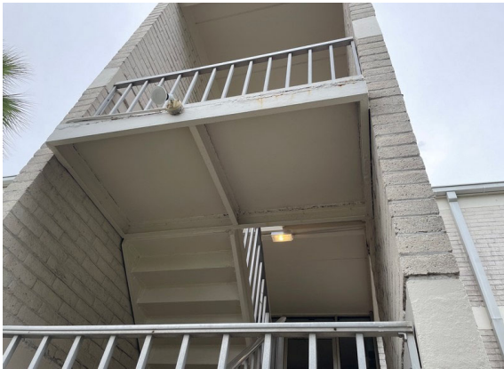
5 stairwell A corrosion
