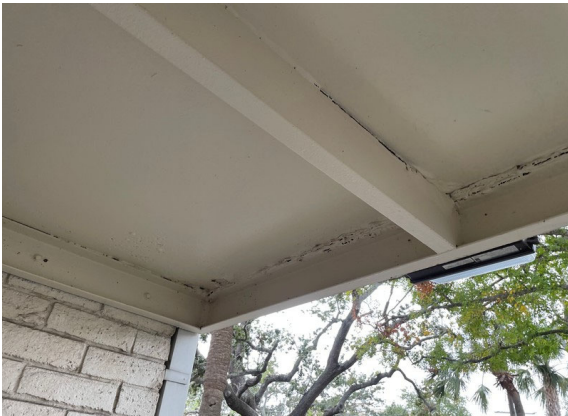
29 stairwell E corrosion
