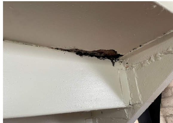
40 stairwell F corrosion
