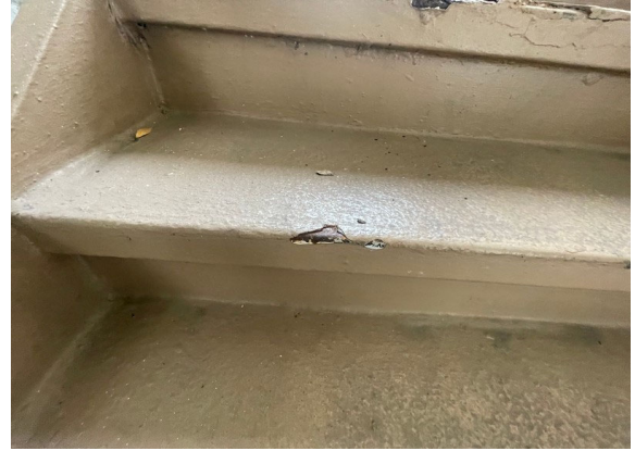
44 stairwell F step corrosion
