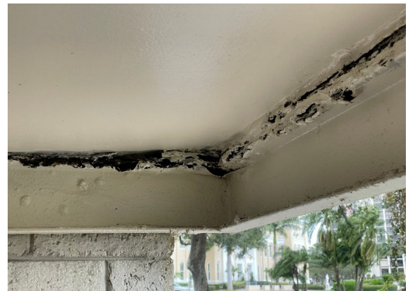
8 stairwell A corrosion
