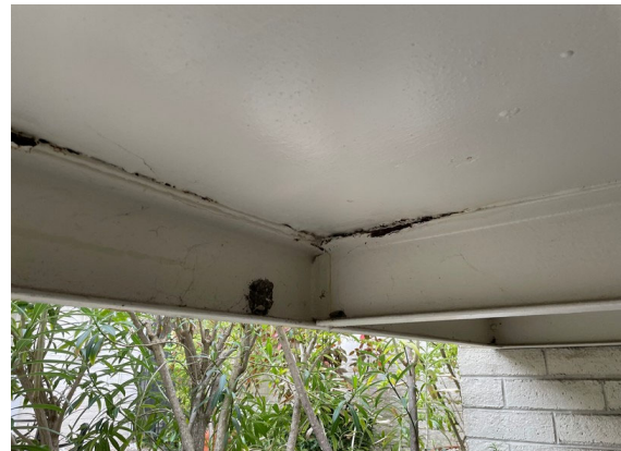
48 Interior stairs corrosion
