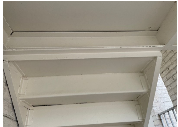
30 stairwell E corrosion
