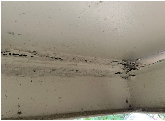
17 stairwell B corrosion
