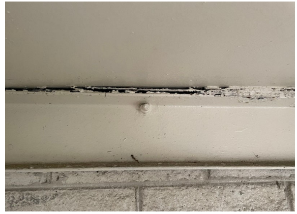
18 stairwell B corrosion
