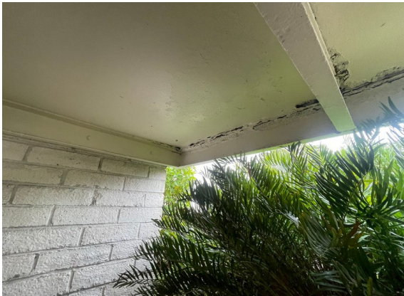
37 stairwell F corrosion
