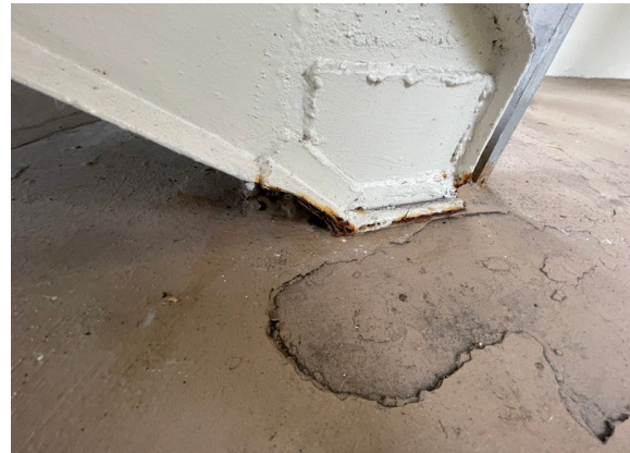
38 stairwell F corrosion
