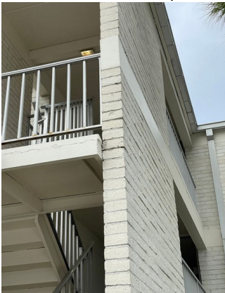
45 stairwell F connection corrosion damaging brick
