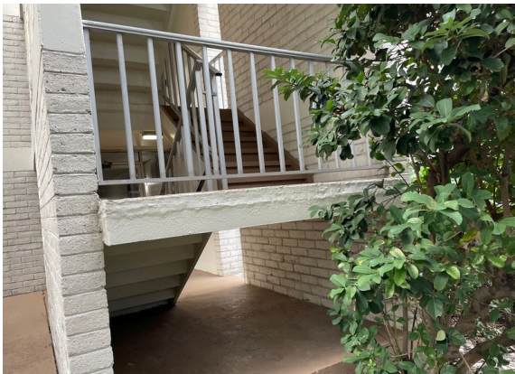
15 stairwell B corrosion
