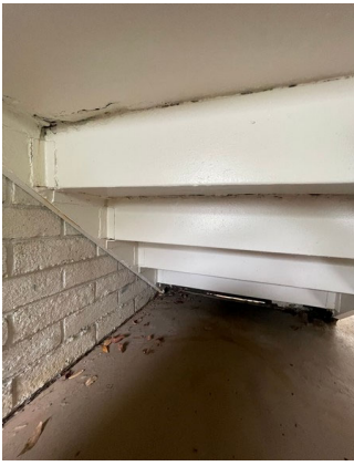
41 stairwell F corrosion
