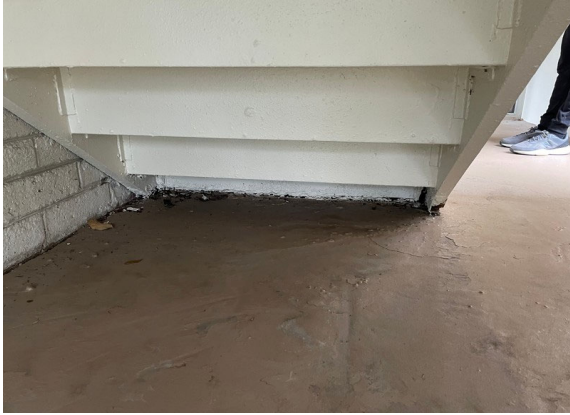
19 stairwell B corrosion
