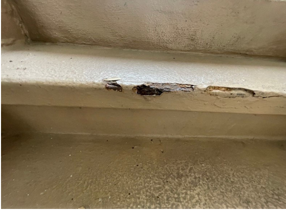
43 stairwell F step corrosion
