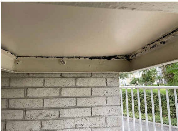
7 stairwell A corrosion
