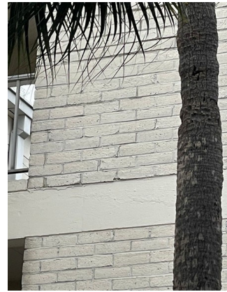
4 stairwell A step cracking in brick
