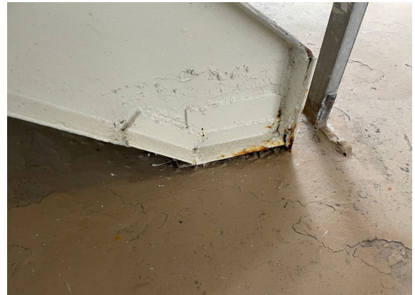
22 stairwell B corrosion
