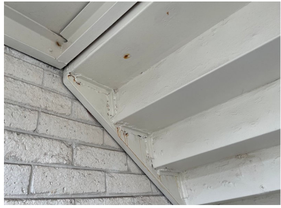
50 Interior stairs corrosion
