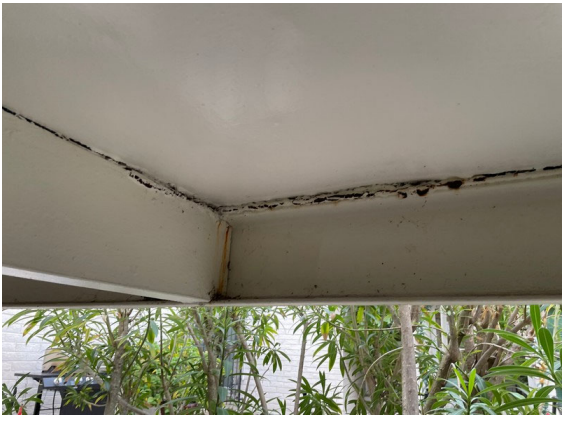
49 Interior stairs corrosion
