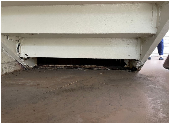
13 stairwell A corrosion
