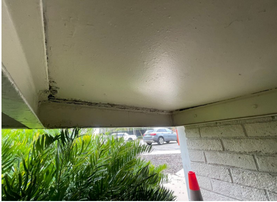
35 stairwell F corrosion
